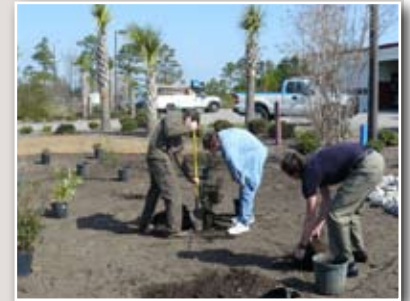
Workshop participants get hands on experience installing a rain garden at the M.B. fire station.
