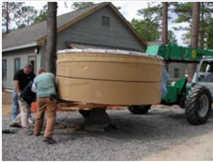
The tank arrives and is carried to an opening left in the building for this purpose.
