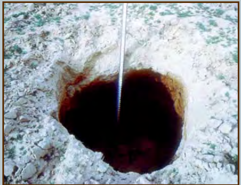
Sinkhole created by the collapse of limestone material just below the surface.
